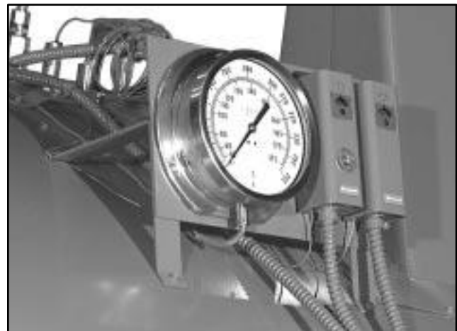
Figure: 6-5 Hot Water Controls
