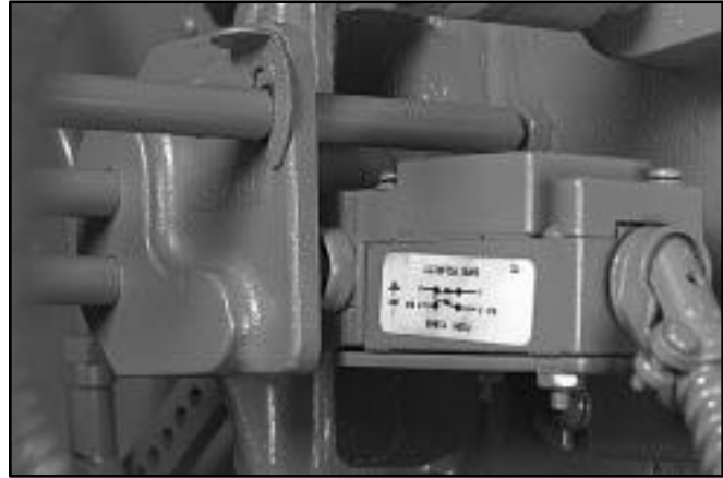
Figure: 6-17 Oil Gun In Place, Oil Draw Switch Closed
