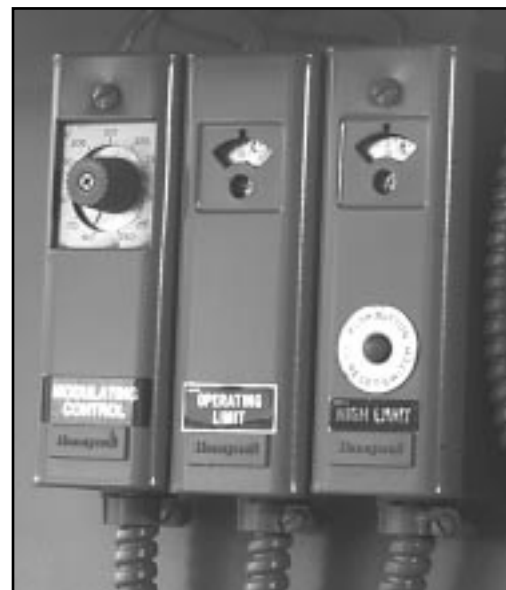
Figure: 6-5 Hot Water Controls
