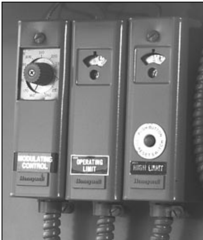
Figure: 1-12 Hot Water Controls
