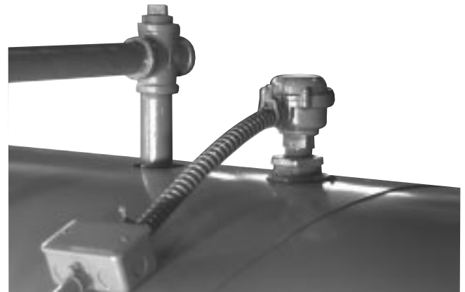
Figure: 1-14 Auxiliary Low-Water Cutoff
